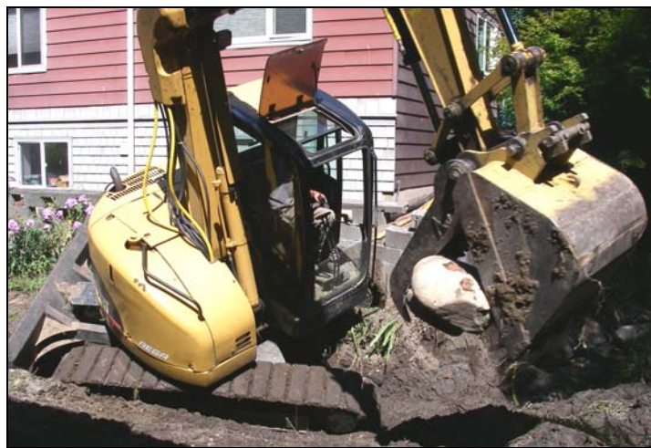
Tight quarters required careful planning and excavating to restore a natural channel without damaging adjacent homes.
