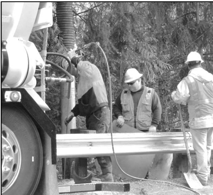
Workers installed more safety guardrail along Marine View Drive SW as a result of FCA and resident advocacy.
