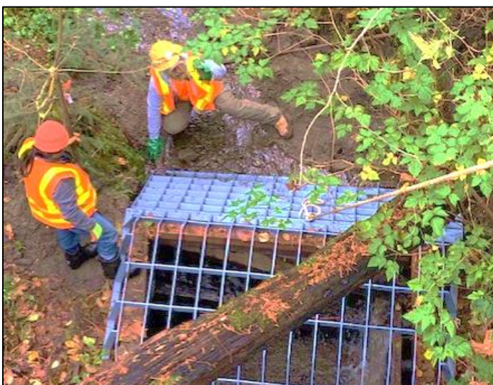
A second grate at the intake should keep large debris out of the culvert under 45th Ave. SW. Photo courtesy Tom Trulin
