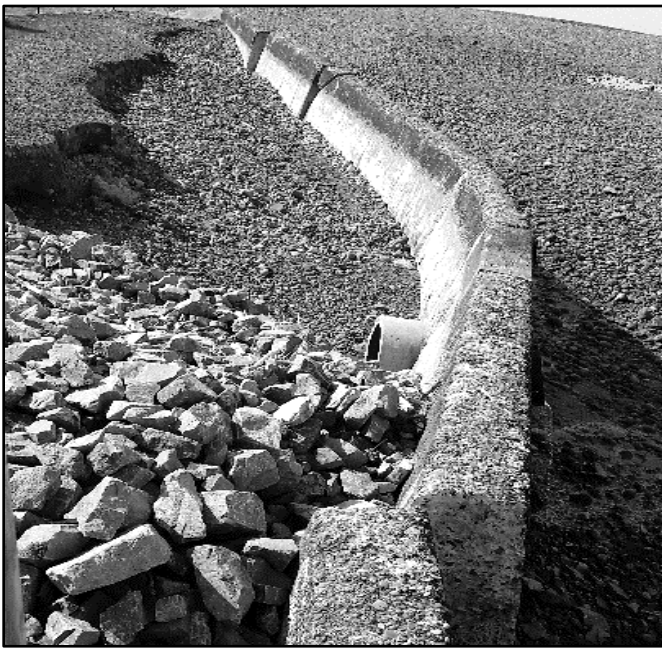
The cracked and tilting seawall at Lowman Beach Park is allowing erosion. Photo courtesy Seattle Parks
