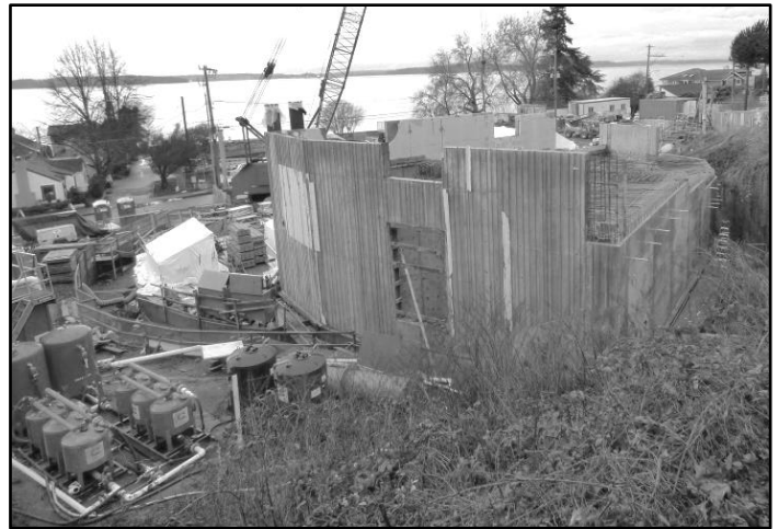
This photo, taken in January by King County Wastewater, shows the building and equipment on the lower left being used to control groundwater while work is under way.
