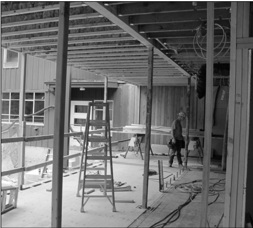
Extension of the church office to the east will gain 10 more feet for staff. (The YMCA wing is in the background.) An enlarged narthex (sanctuary lobby) below the office, with a patio, will be open to the view into Fauntleroy Park. Photo courtesy Phil Sweetland
